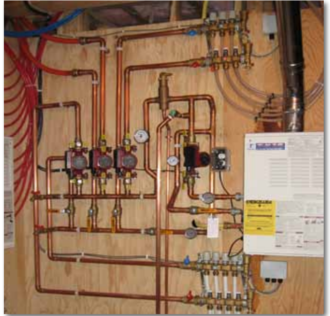
A complex system of zone valve solenoids, primary loop circulation pump and zone circulation pumps shown here are easily monitored by InduSoft Web Studio.
